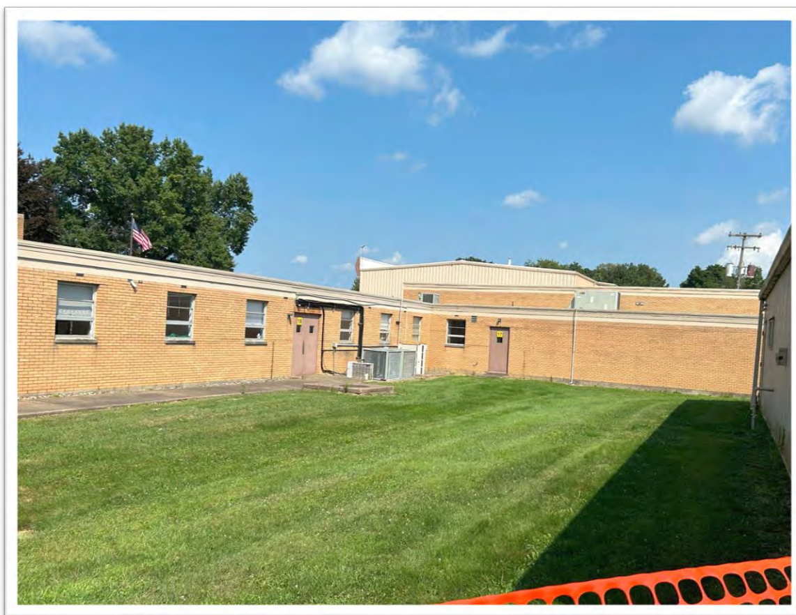
Figure 5: Photo of the alcove and A/C unit by which Crooks gained access to the AGR roof 246
